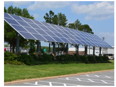
Ground-mounted solar panels.
